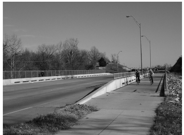
Figure 5. The same location in 2008, after highway improvements were carried out according to the 2004 street design standards
